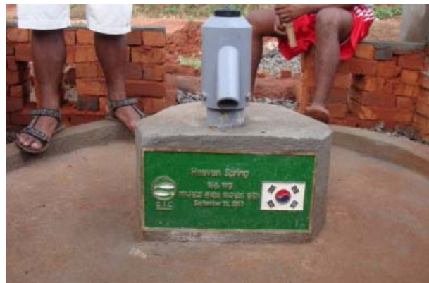
Figure 4: Water point with hand pump and concrete slab
